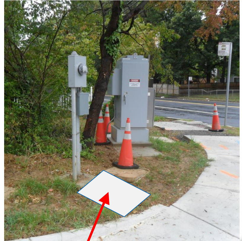
Electrical service work pad needed
